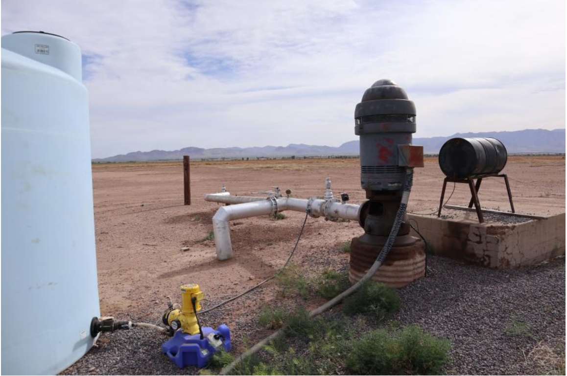
Turbine pump, 150 Hp, electric, D4 pivot
