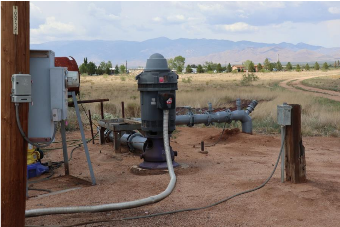
Turbine pump, 150 Hp electric, C1 pivot
