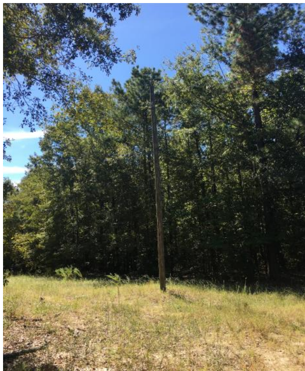
Power on Site
