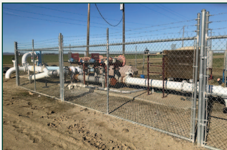
Filter System (1 for each block)
