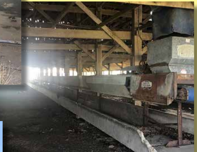
180' belt feeder trough
