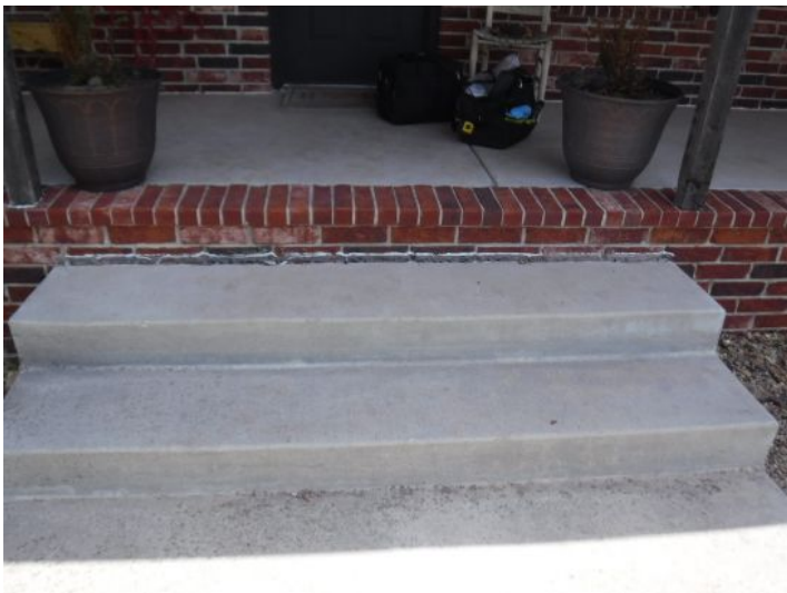
The front steps have settled
