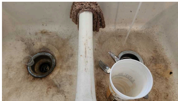
Stains noted in the Kitchen sink
