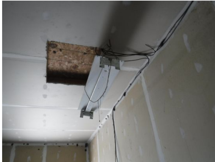
OSB covers for attic access are not a fire rated material
