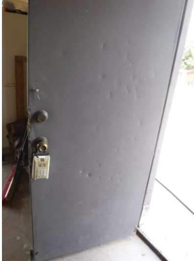
The East exterior door from the garage has some dents
