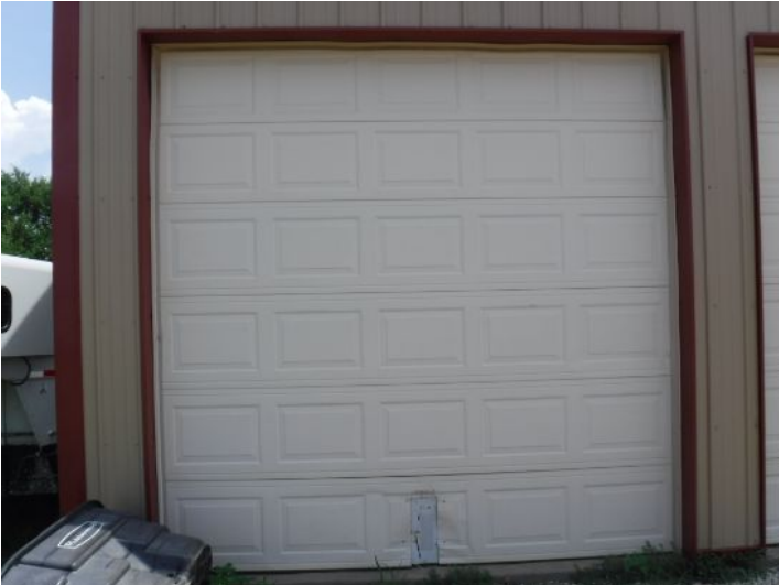
Damage noted on the lower door panels
