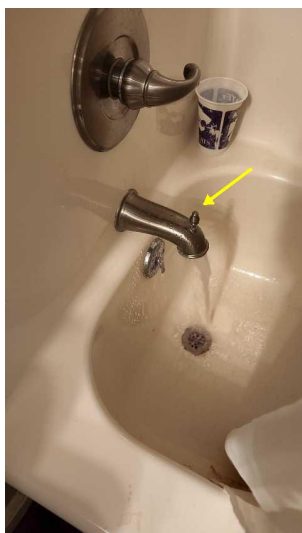
Diverter does not seal properly
