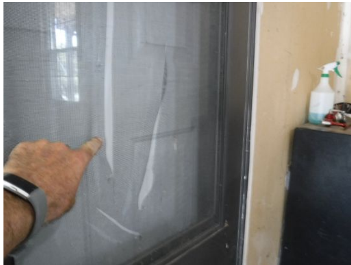
Frayed screens noted
