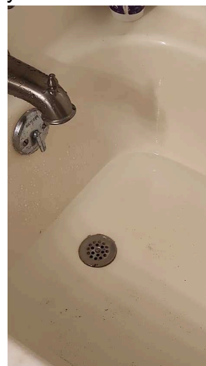
The Main floor bathroom tub drains slowly. Recommend cleaning.
