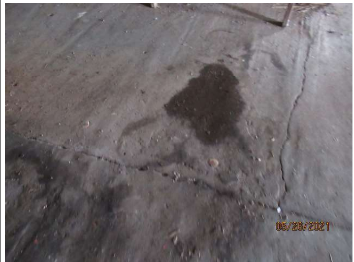
Stained concrete inside the vacant shop.
