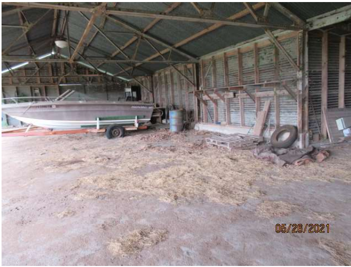
Boat and debris observed beneath overhead shed.
