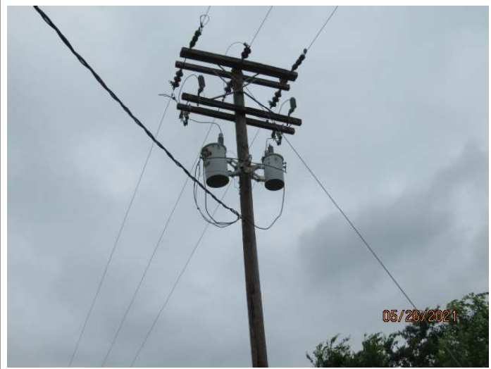
Electric transformers observed near feed lot corral.
