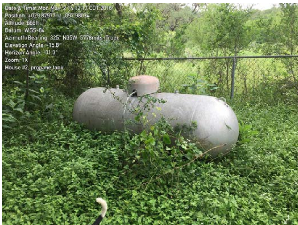
Photo 14. House #2, propane tank
