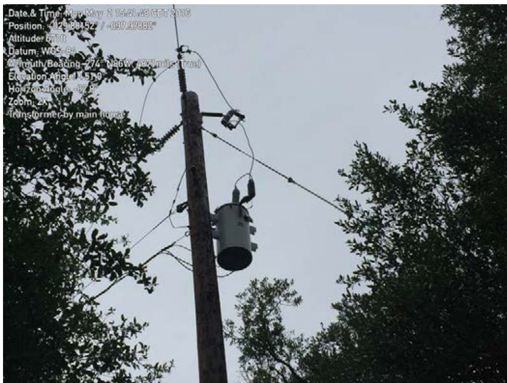
Photo 20. Transformer by main house
