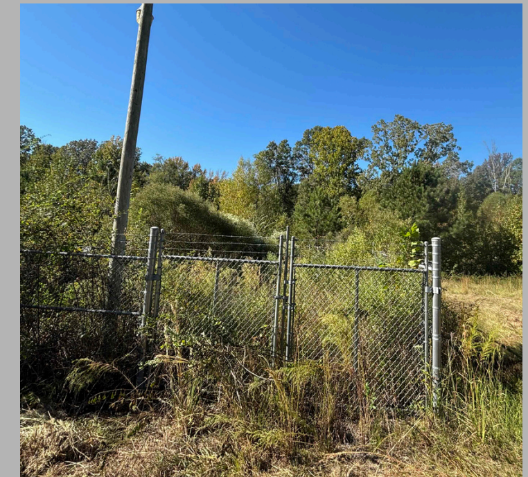
Commercial Sewage Lift Station
