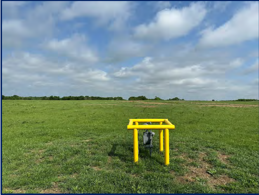
Atmos Pipeline-Texas pipeline meter with barricade.
