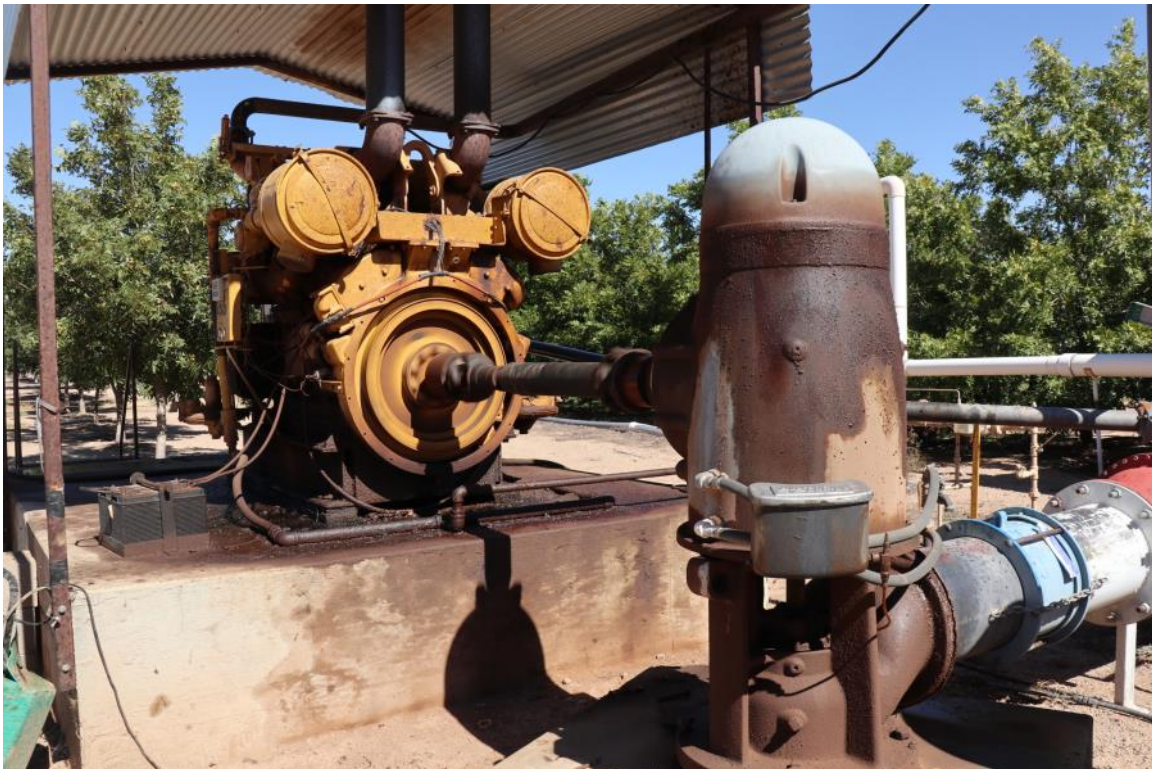
700' well, Cat natural gas engine, 1,500 GPM
